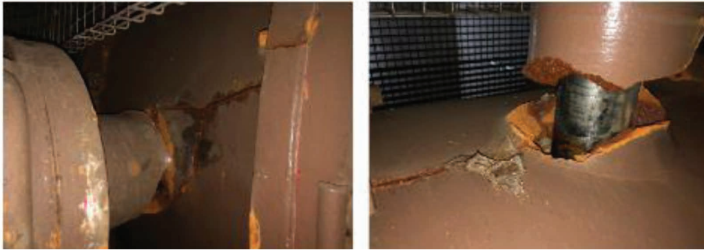
Damaged butterfly valve at Driekoppies Dam inlet
