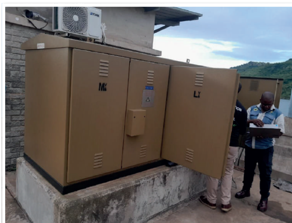
The sub-station that has been installed at Maguga Dam tower.
