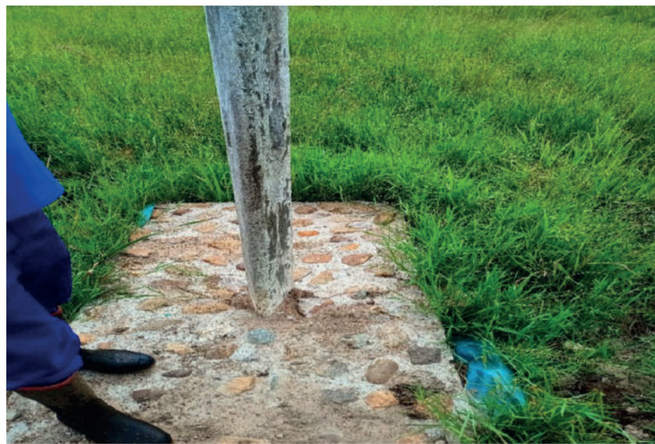
Weekly inspection of the mud boils.
