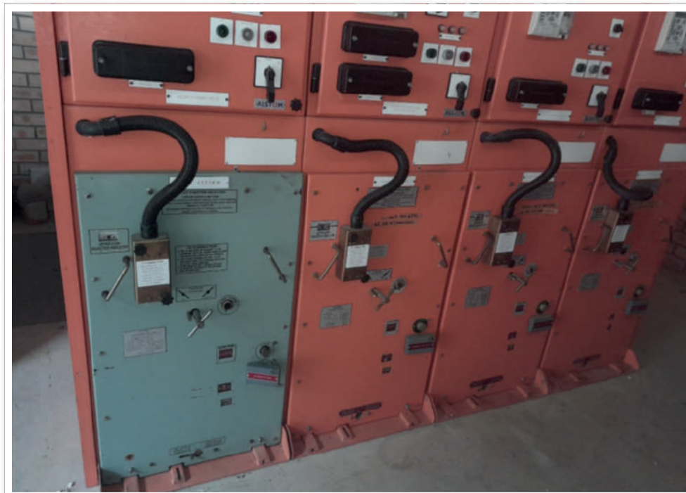
The recently installed switchgear at the incomer.
